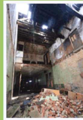
Walnut Hills Redevelopment Foundation is taking on the firehouse on McMillan. Years of neglect have collapsed the roof and second floor!
